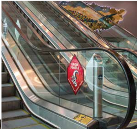
A Escalators Glass Panels
